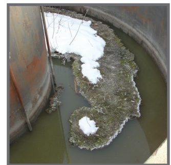
Large sewage raft from equalization basin
