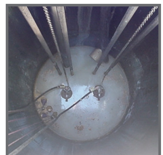
SH PUMPS IN WK NORTH MEDICAL CENTER WET WELL
