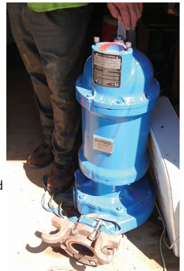
4XSH PUMP AT PHYL BEN VILLAGE LIFT STATION
