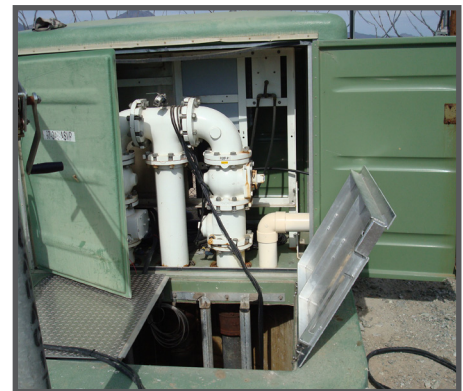
GILA RIVER INDIAN RESERVATION LIFT STATION 2
