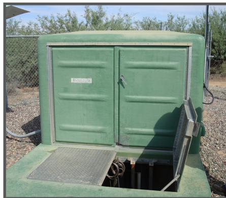
GILA RIVER INDIAN RESERVATION LIFT STATION 1
